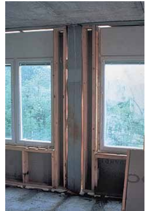
1.17 Integration of a steel column in a timber framed façade (covered with gypsum board on the inner side). Without additional measures, the fire resistance of the column is at least 30 minutes.
