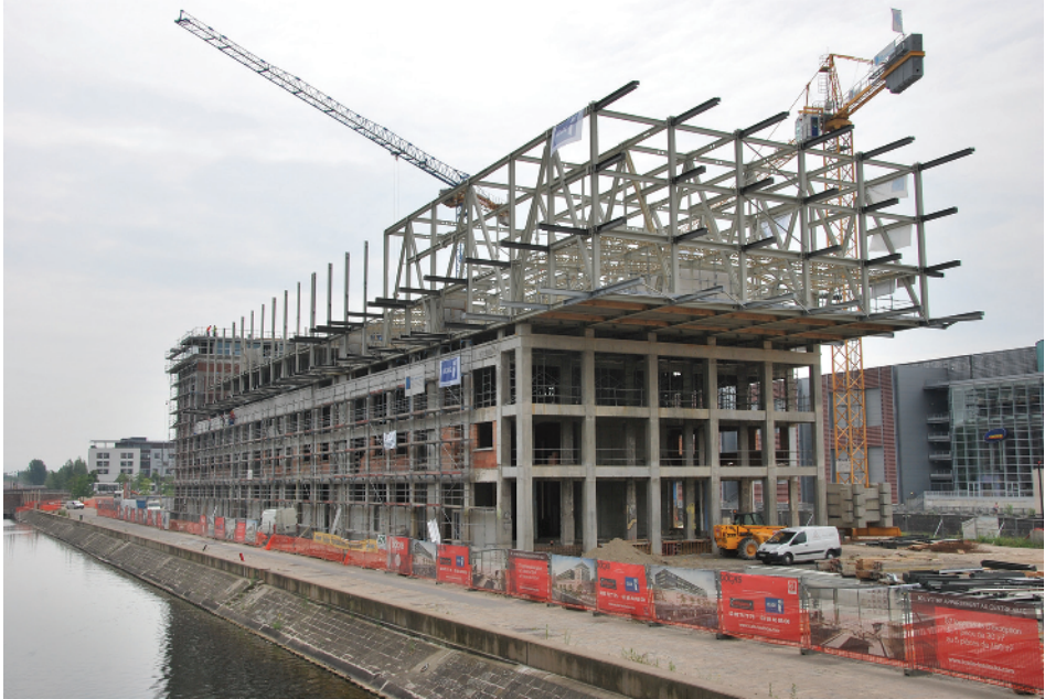
Figure 2 The old Seegmuller warehouse, built in 1932, was refurbished and enlarged by a three-storey steel structure. © ConstruirAcier.
